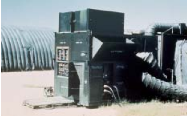
Fig. 6-5. The mechanical equipment used to operate a MUST (medical unit, self-contained, transportable) hospital consisted of a gas turbine, a generator, and an air-cooling unit, which together constituted a utility pack. Large tubes acted as conduits to provide cooled or heated air to the treatment areas.
